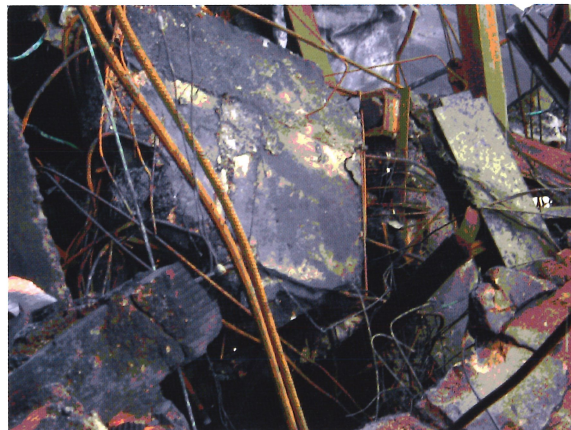
Figura 13. Restos de pilar de hormigón colapsado Figure 13. Remains of a collapsed concrete column
