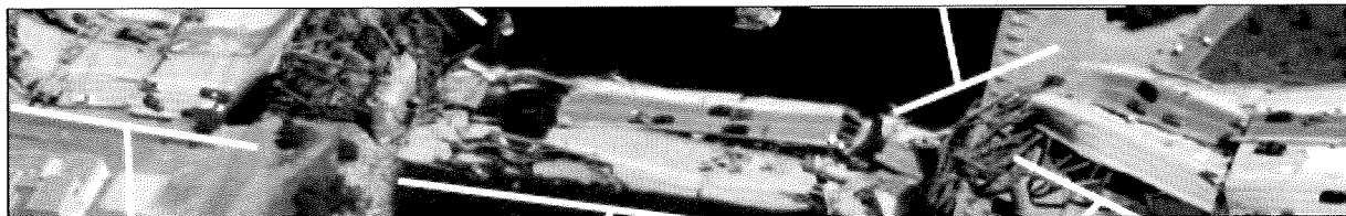
Photograph 36. Bridge on I-35W at Minneapolis, USA. Overview of bridge after collapse Fotografía 36. Puente de Minneapolis (USA). Vista general del puente colapsado
