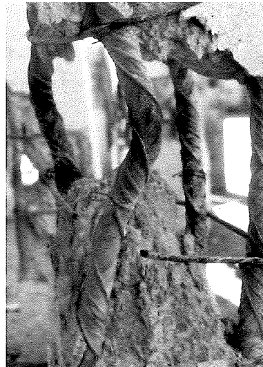
Figure 4 Effect of transverse reinforcement in columns with high steel ratios (INTEMAC tests, 1972) (6)
