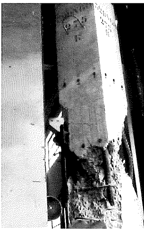
Figure 5 Column fracture, standard stirrup distribution (INTEMAC tests, 1972)
