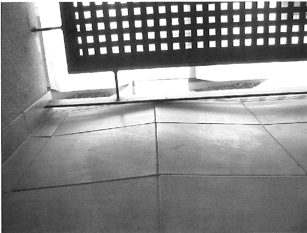
Figure 7. Loose, upward slanting tile.
