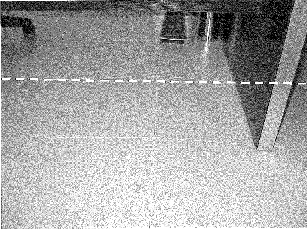
Figure 8. Loose, upward slanting tile in interiors.
