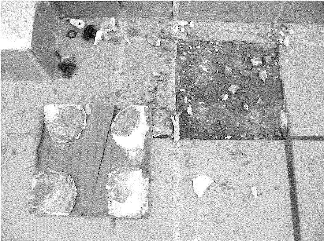
Figure 14. Detachment of porcelain tile due to irregular application of the adhesive ("towel lumps" on the back of the tile).
