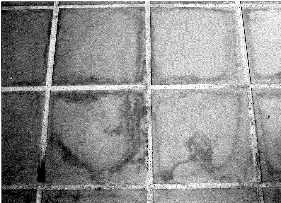
Figure 16. Stains on ceramic tile laid on an outdoor waterproof surface.
