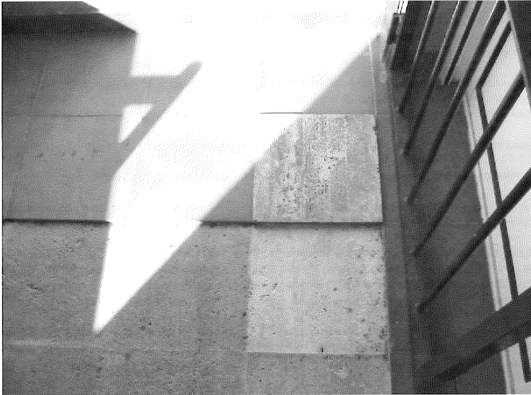
Figure 6. Detached tile on outdoor flooring.
