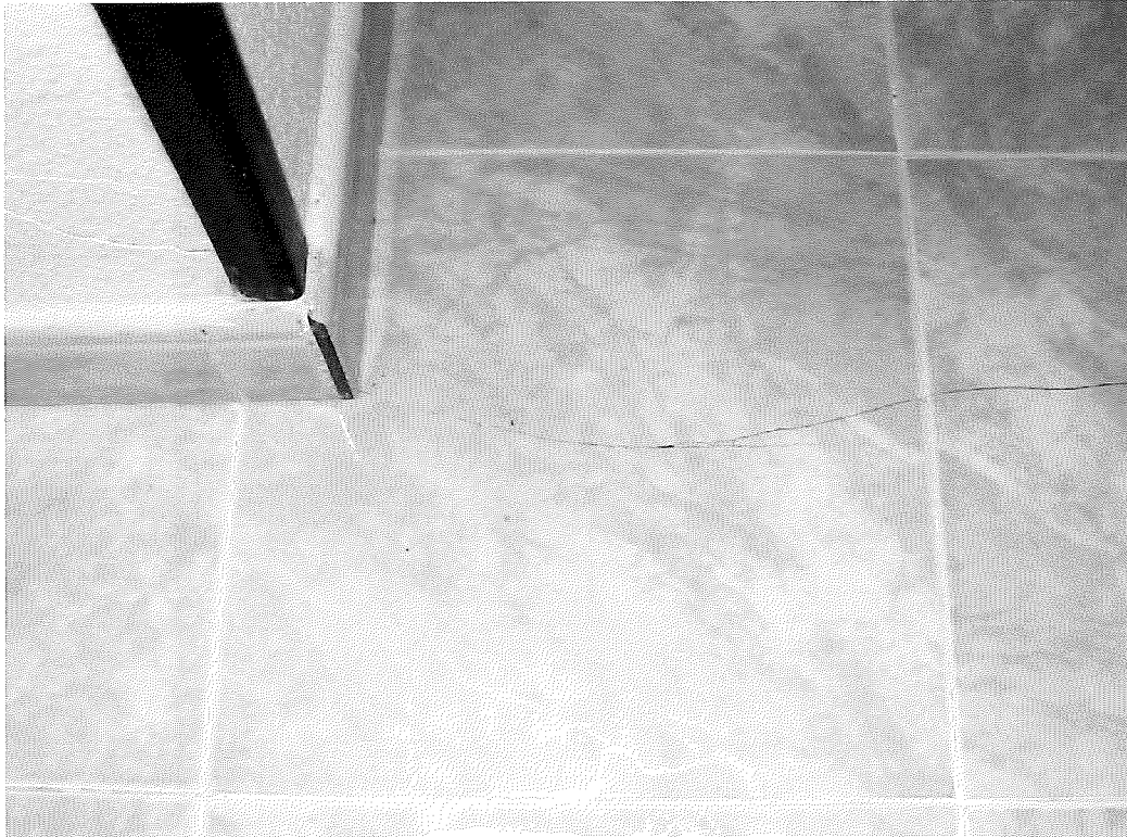
Figure 3. Cracks in flooring due to excessive slab deformation (note that the wall on the left is also cracked).
