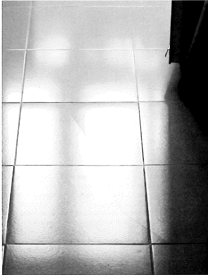
Figure 1. "Waves" (top) and closed cracks (bottom).
