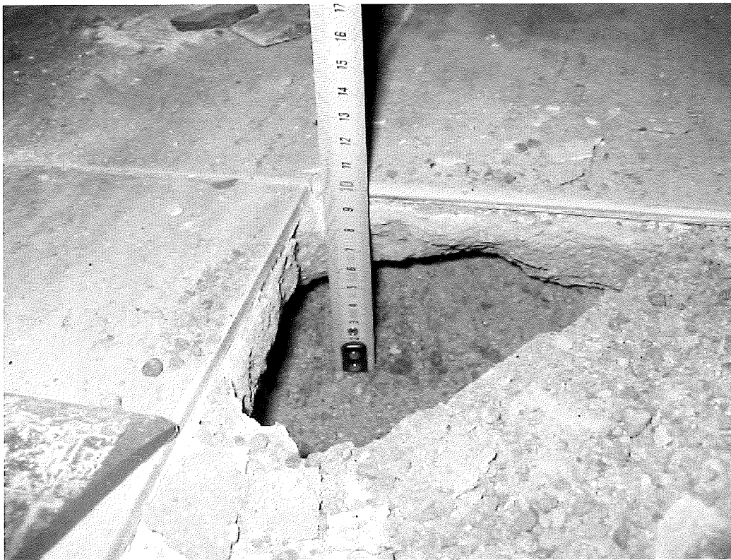
Figure 4. Measuring the thickness of the sand layer (6 cm) in a cracked tile floor (note also the irregular grain size distribution of the sand)
