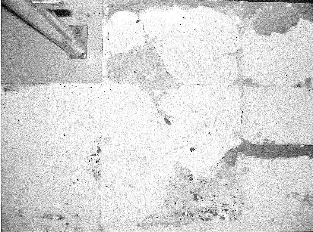
Figure 13. Detachment of porcelain tiles due to irregular application of the adhesive (white material) and placement after the "open time" had lapsed.
