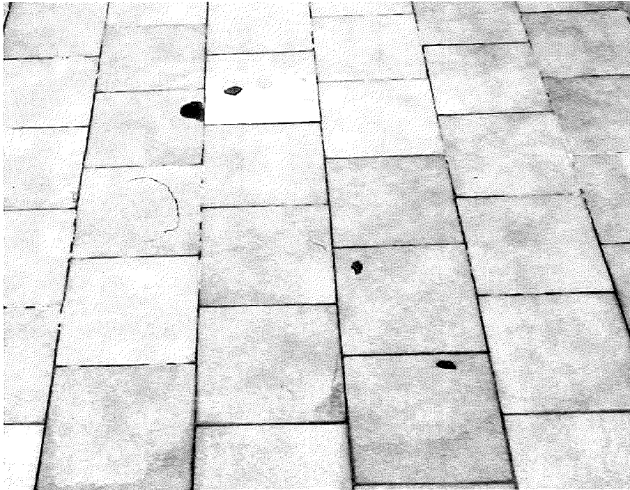
Figure 15. Chipped ceramic tile laid on a waterproof outdoor balcony.
