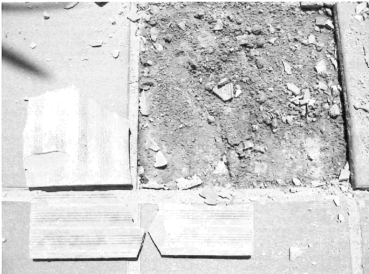
Figure 5. Detachment of a low absorption porcelain tile in an outdoor location, received in cement mortar (note that there is no mortar adhered to the back of the tile).
