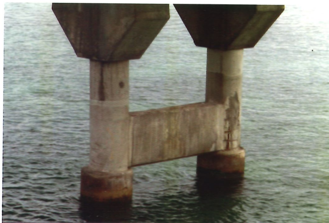
Figure 8: Bridges on the Florida Keys: Critical damage of piers due to corrosion of epoxy coated reinforcement.
