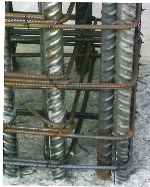
Figure 10: Two pictures illustrating the combination of stainless steel reinforcement and ordinary black steel reinforcement. Above only the deck part later to be exposed to a marine environment is SSR. To the right a shift in the two types of reinforcement is made in a column at a height where chlorides from the environment are no longer expected to enter the concrete
