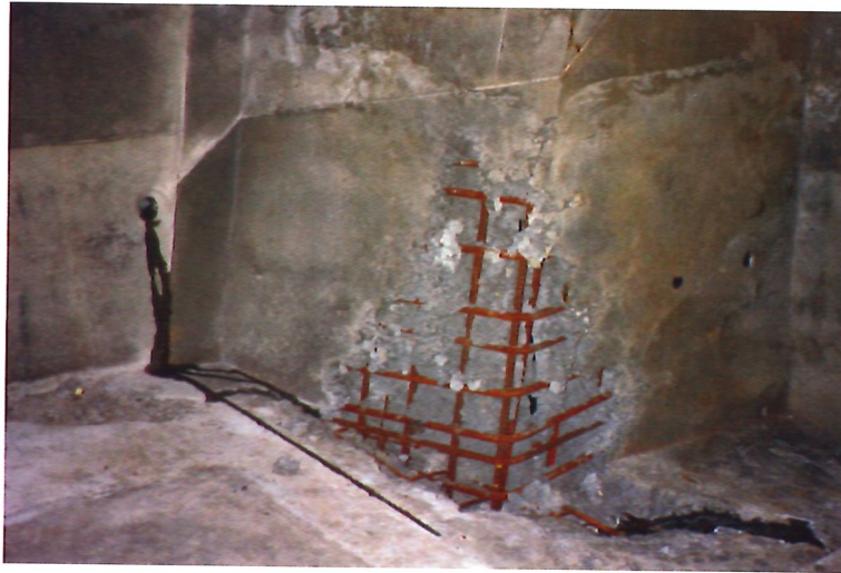
Figure 2: Typical honeycombing in a new construction. Such execution defects leads to repairs of most large scale new concrete structures.
