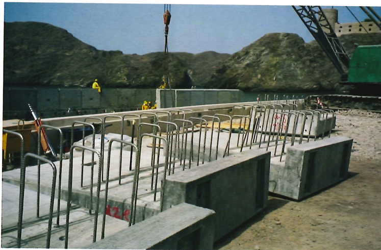
Figure 15: Stainless steel reinforcement used in the precast structural members to replace a corrosion damaged seawall protecting the Palace and the new Guest Palace Complex (Figure 14) from the Gulf of Oman.
