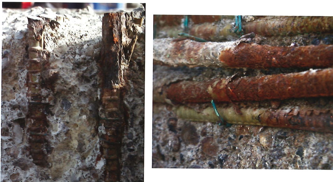
Figure 9: Two pictures illustrating the adverse corrosion protection performance of epoxy coated reinforcement in the vicinity of the saline waters of the Arabic or Persian Gulf under hot and humid environments.
