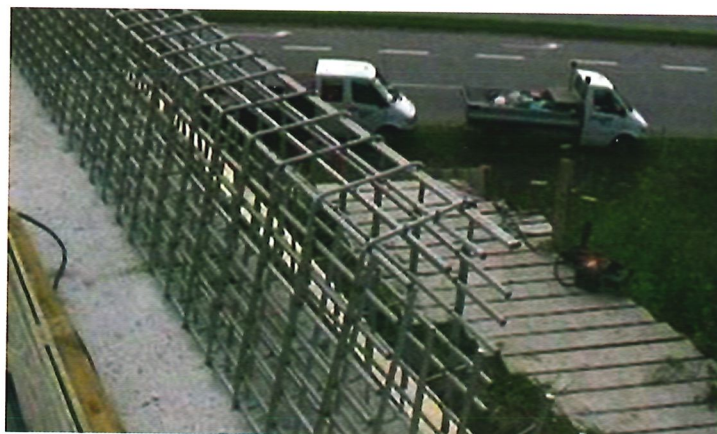
Figure 16: Replacing edge beams and parapets on bridges in Denmark exposed to de-icing salt. Stainless steel reinforcement is introduced to avoid future repairs causing major traffic disturbances. Also new structures are being provided with stainless reinforcement in the edge beams and parapets as they are highly exposed to de-icing salts during winters.
