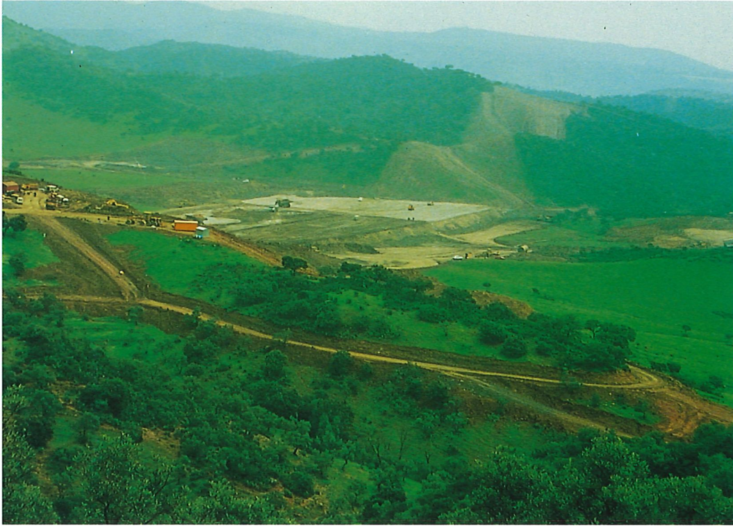
1-Vista general al comienzo del relleno. General view on the commencement of work.
