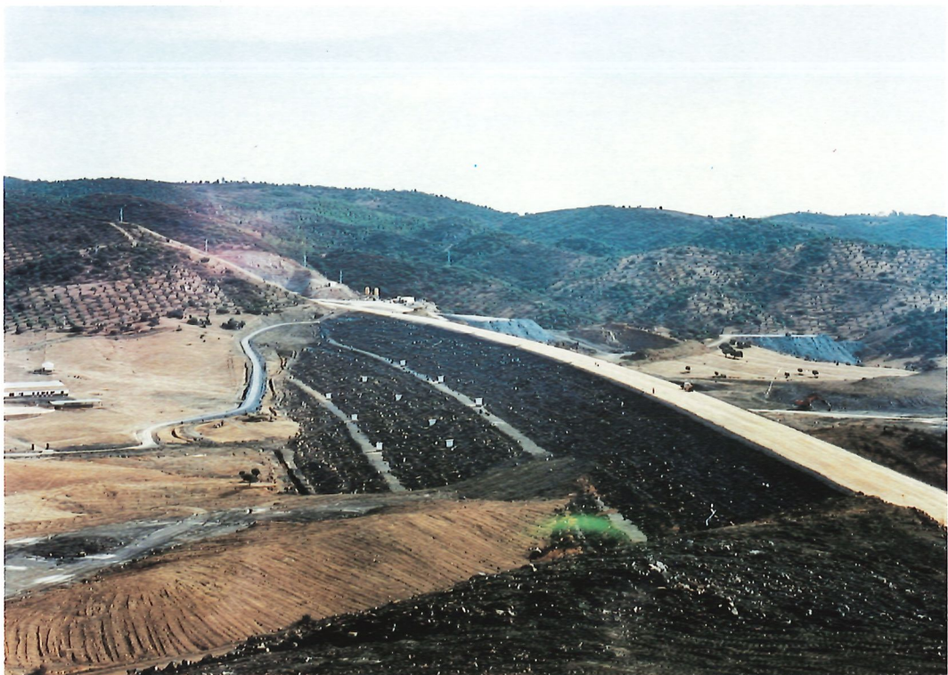
4-Relleno acabado, a falta de subbalasto y balasto. Finished backfill, awaiting subballast and ballast.
