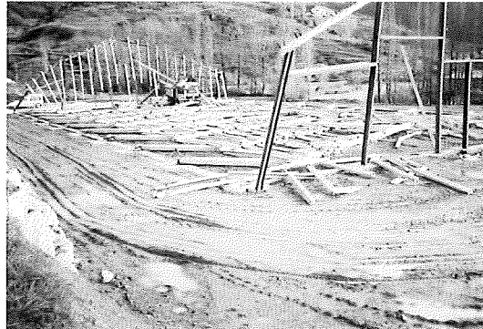
Hundimiento de una nave no suficientemente arriostrada durante su montaje Collapse of an industrial bay during construction due to insufficient shoring Fig. 27
