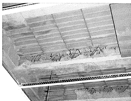
Defectos de hormigonado en un forjado de viguetas semirresistentes Concreting flaws in a slab with non-self-supporting joists
