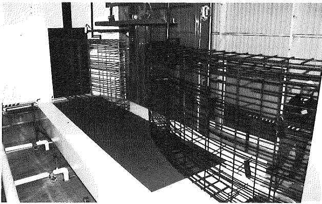
Fig. 16. Fluidized bed dipping technique used for epoxy coating of 3-D fully welded, grit basted and pre-heated reinforcement cages.
