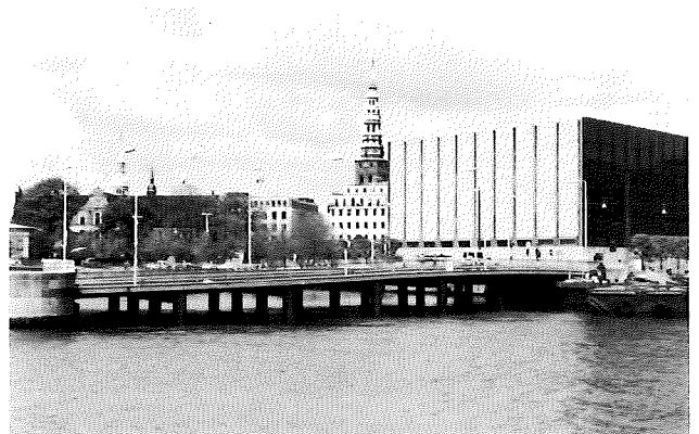
Fig. 15. Stainless steel lined column in saline waters.
